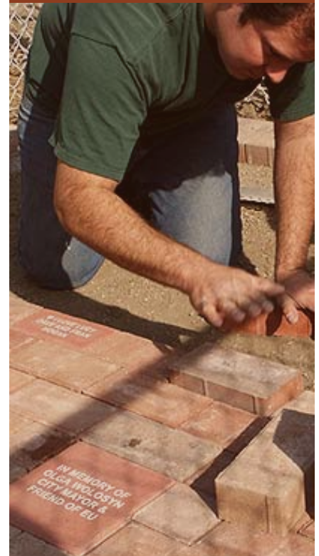
Tavis Hanna installs bricks at the Canine Corral between the two west gates.
